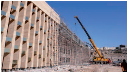
Construction work at the new museum in winter 2013 (Photo, top: NB, bottom: MA).
