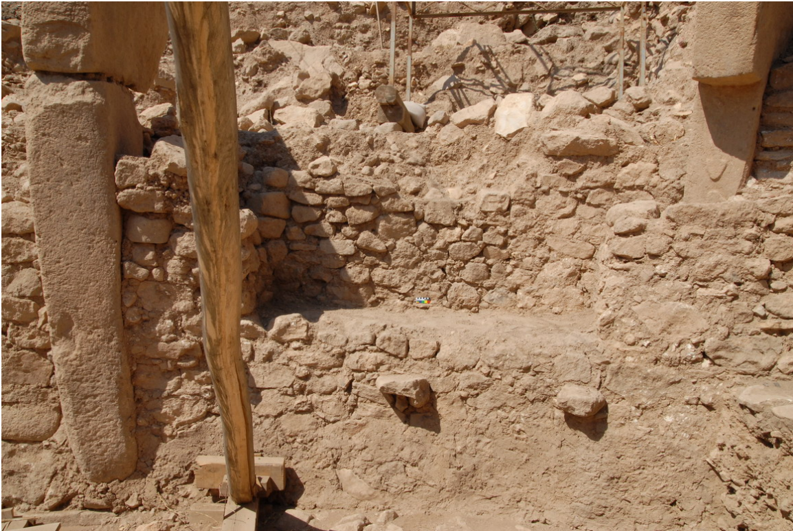
Above: Daubed plaster lower wall with damage to wall above.
