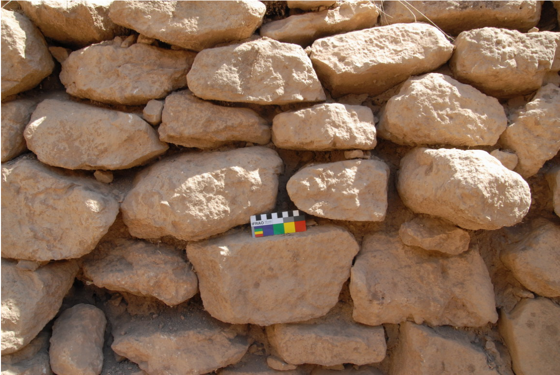
Above: Detail of wall with eroded pointing, excavated in 2005.
